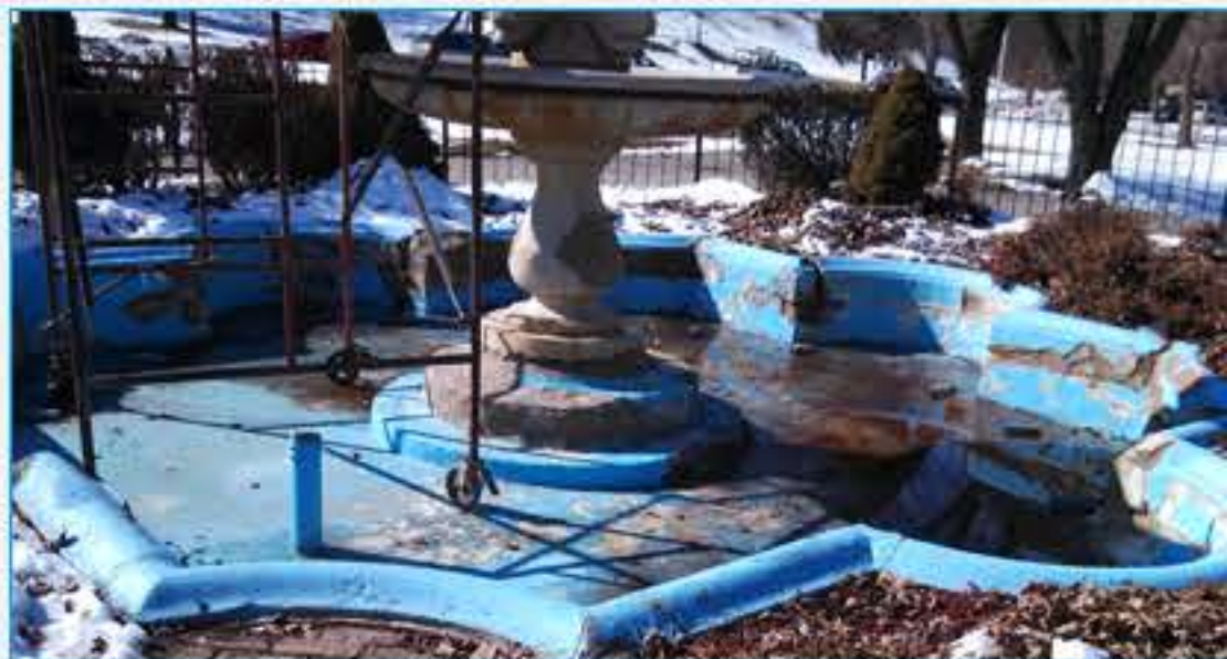
Civic Center Fountain before repairs
