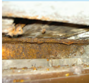
Rusted lintel that could be improved with Tuckpointing
