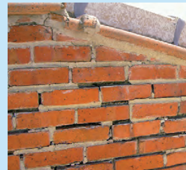
Example of bricks needing Tuckpointing
