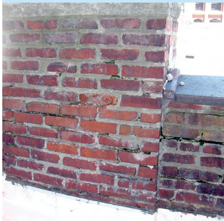
Example of bricks needing Tuckpointing
